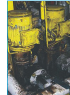
Leakage on pumps with mechanical sealing
