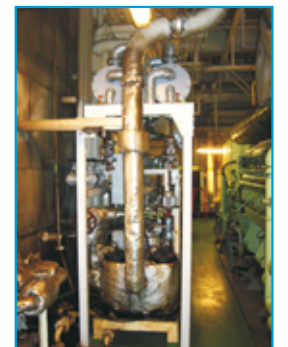
After: with new shell & tube heaters
