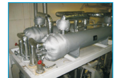
New installation: 2 shell & tube heaters
